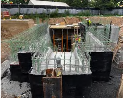
Backfilling along the Main Entrance staircase and Escalator foundation walls has progressed.
