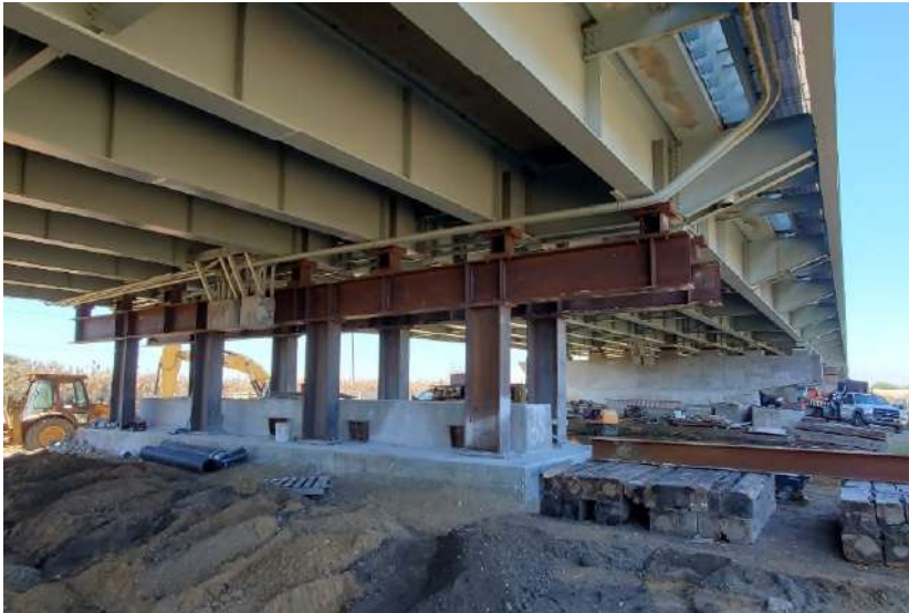
Temporary steel supports installed. The supports raised the bridge 1/8” to allow removal and installing of a new concrete pier.
