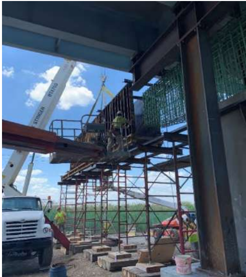
Crews construct concrete forms in preparation of pouring the new concrete pier.
